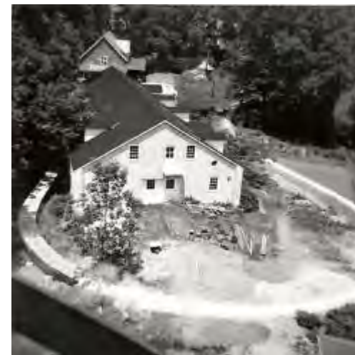
Ongoing construction of the Auburn Valley Railroad, 1960. The Marshalls hired Everett Hollingsworth of Fairville, Pennsylvania, to lay out, build, and grade the roadbed for a loop around the Auburn Heights property.
